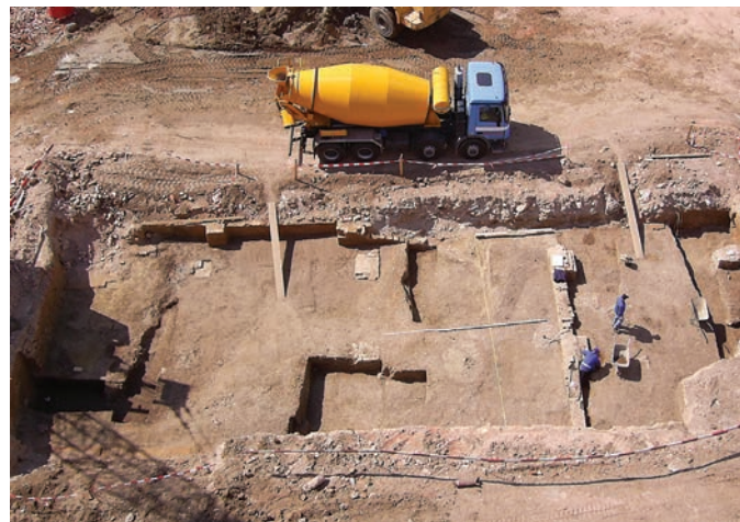
145. There is a constant need for the town archaeology in Vienna to document Roman remains before they are overbuilt or removed
